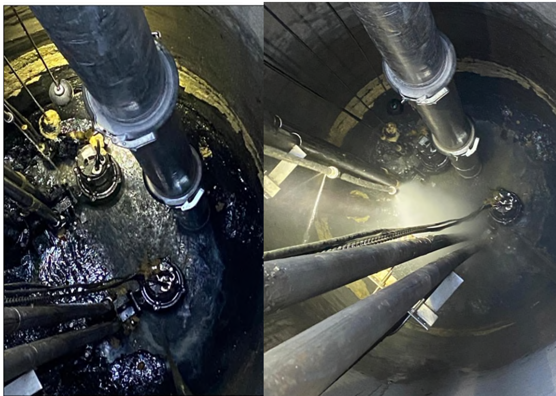
STATION 4 SCHEDULED FOR REPAIR OF BOTTEN OF WELL SEPARATING
